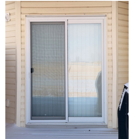
Back Patio Doors
